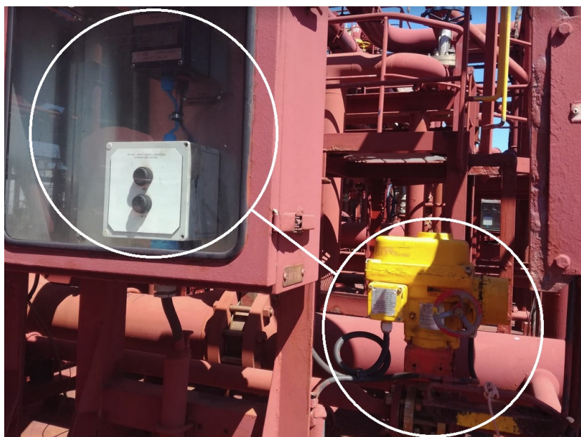
Fig. 4. An automatic valve before Ethylene vaporizer
