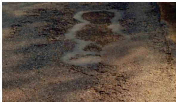
Fig. 7. Surface aggregate and binder losses [13]
