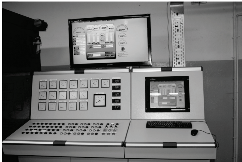
Fig. 2. EMOS working station
