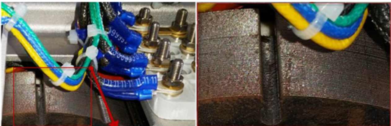
Fig. 3. Laminated stator core of the brushless synchronous generator exciter
