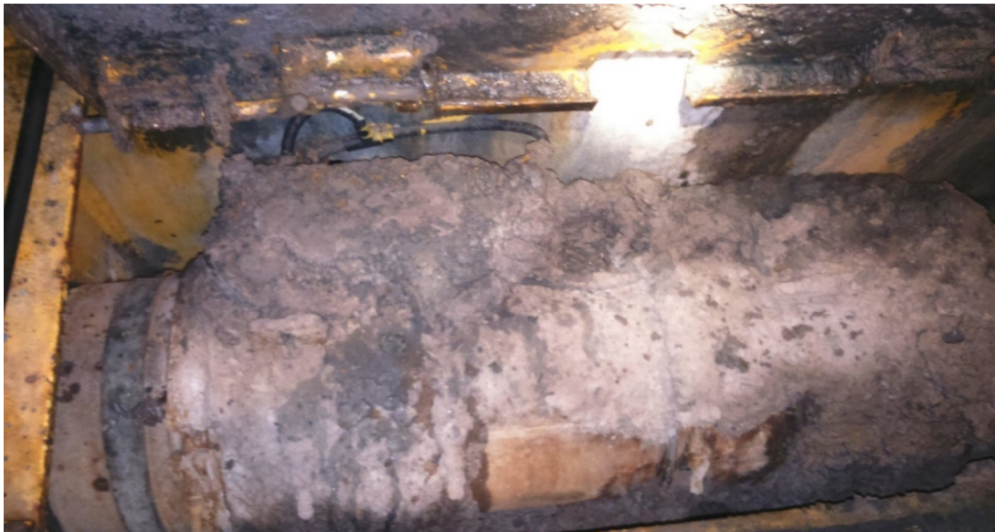
Fig. 4. Engine No. 2 – view of the particulate filter
