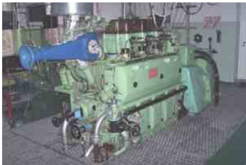
Fig. 1. General view of the Sulzer 3 AL 25/30
